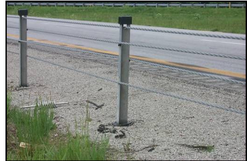
Figure 17. I-71 Cable Barrier
